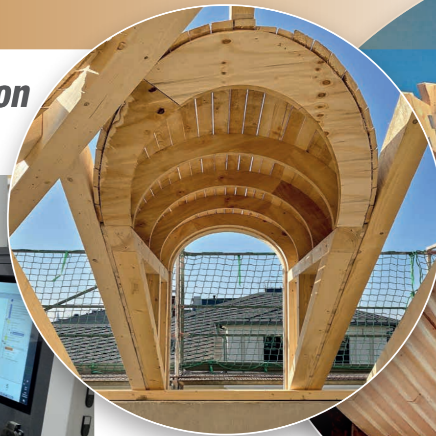
Dormer window construction: 70 dormer windows were required for the roof truss of the Königshöfe Dresden building project.
